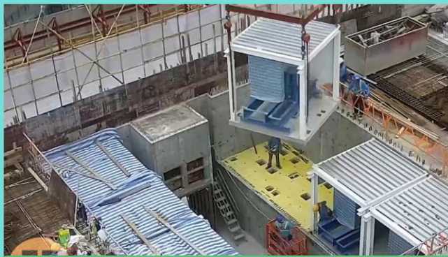
MiC Lift Machine Room
